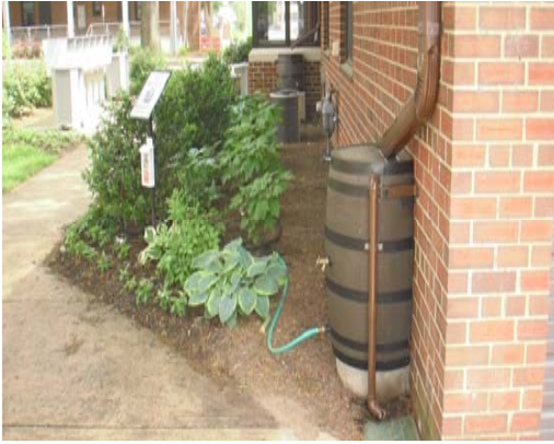
Installation at the Hightstown Housing Authority with soaker hoses attached to water the gardens.
