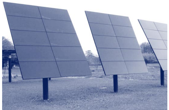
Ground-mounted solar array
