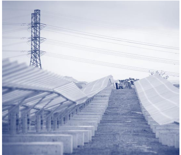
The first state-owned landfill solar farm in Kearny, NJ Governor’s Office/Tim Larsen
