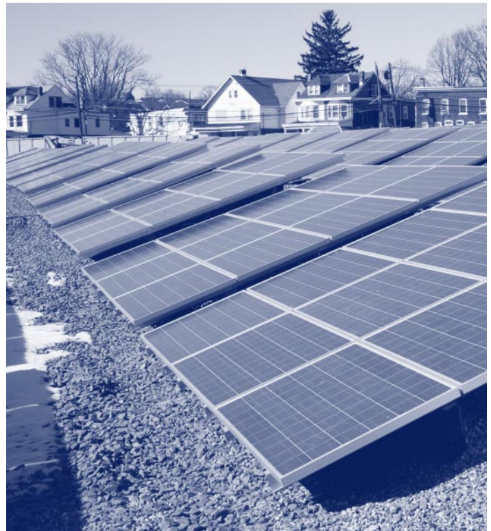
A ballast system was used to anchor the solar panels on this 1.3 MW PSE&G facility on a brownfield site in Trenton, NJ. Peter Craig
