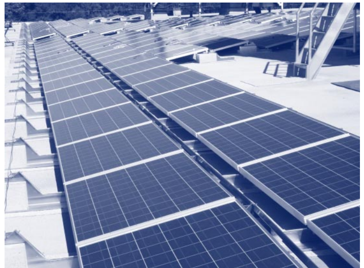
Roof-mounted solar panels at Mennen Sports Arena in Morristown, NJ
