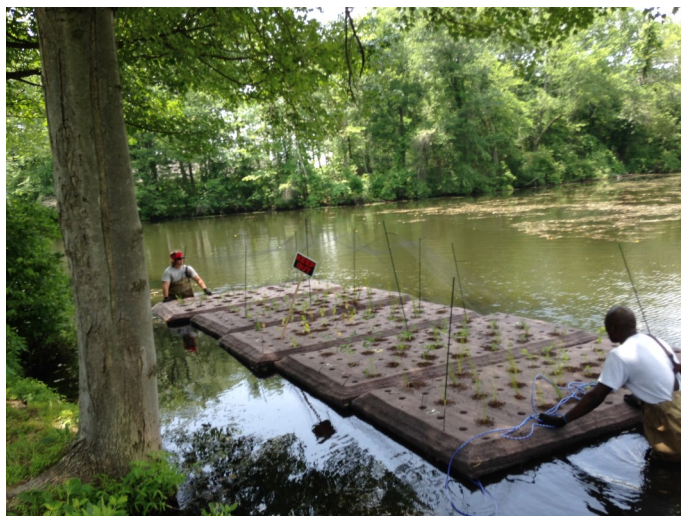
Installation of floating wetland islands at Ashley Cove in July 2014 at Lake Hopatcong
