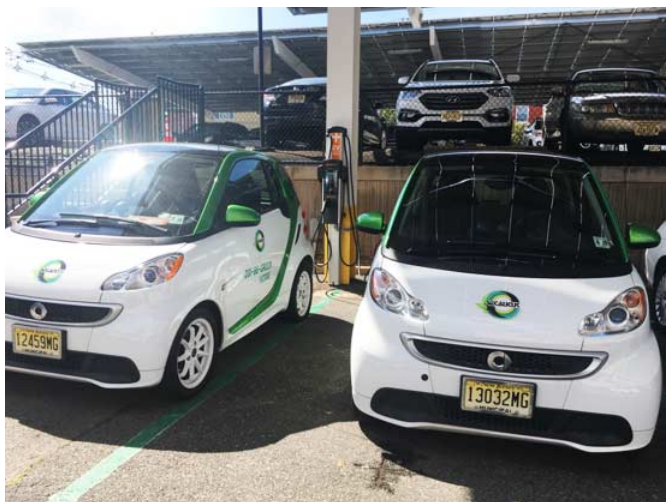
EV charging station in Secaucus
