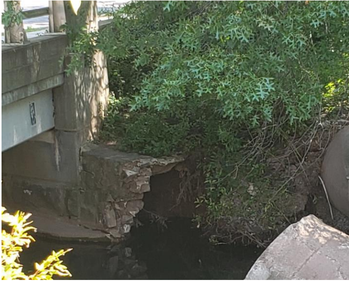
Stream Erosion and Undermining at Oakland Road
