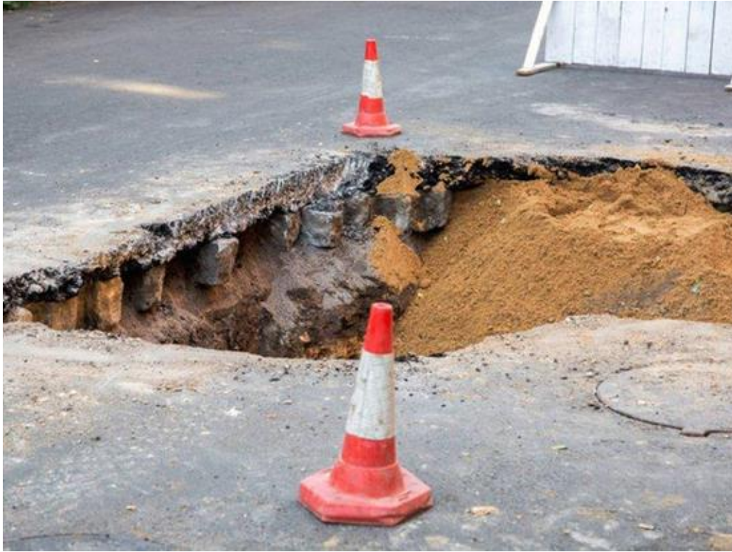
New Brunswick (George Street) 34-foot sinkhole caused by record precipitation overwhelming a culverted stream, 2018
